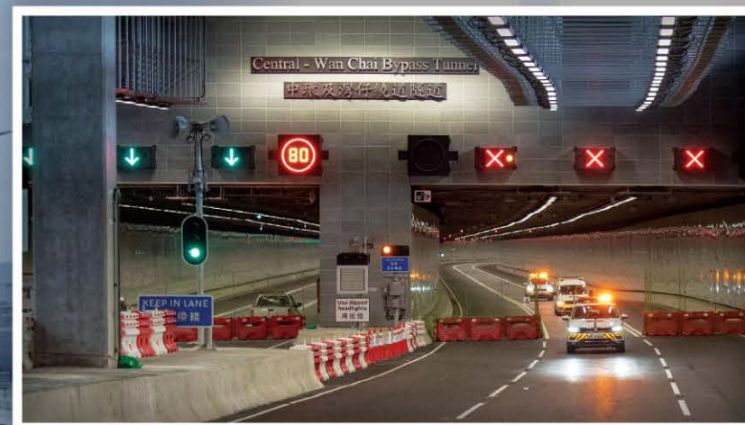
TL Central - Wan Chai Bypass - Schreder FV33xp Tunnel Light
