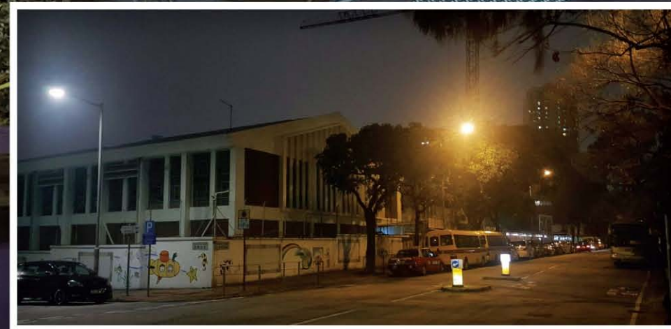
SP Kowloon City - Wireless Lighting Control System
